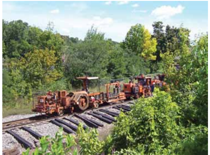
Norfolk Southern track crews replacing ties, smoothing the track and improving grade crossings between Ypsilanti and Kalamazoo.
