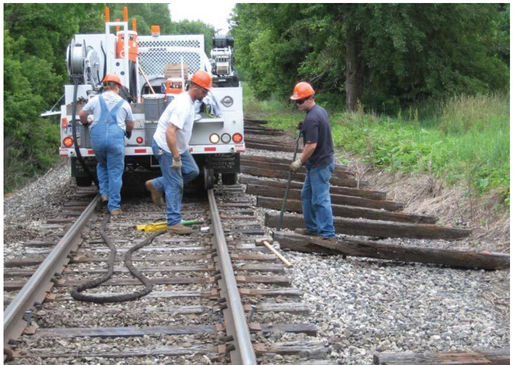
Maintenance track team replacing ties in major infrastructure rehabilitation of the Grand Elk Railroad in 2009. The railroad will have replaced 15,000 ties by the end of the year substantially improving rail service across the entire line.
